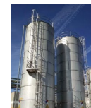
CARBON AND STAINLESS STEEL TANKS
